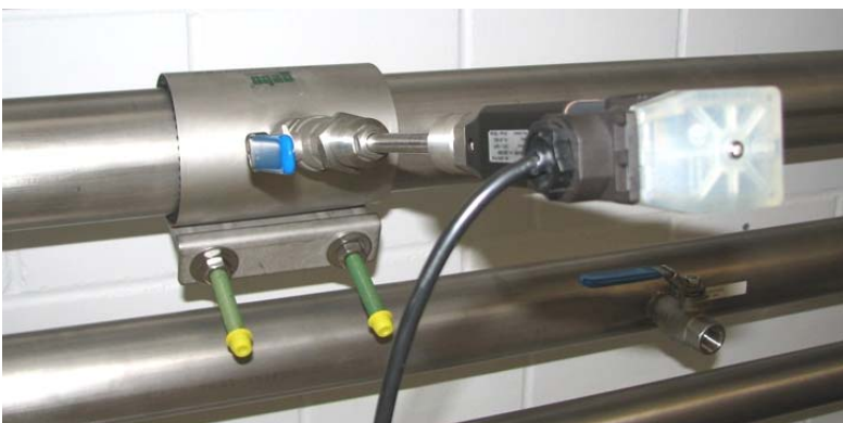
Example: VA 300 flow and consumption measurement
