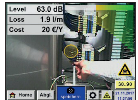
Leaking plug connection
